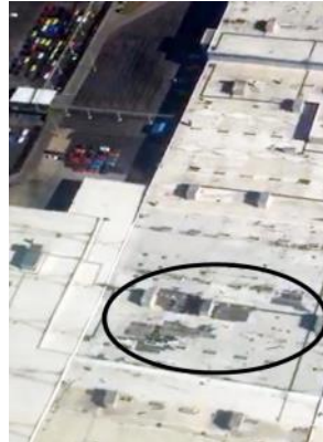
The hole in the roof of the Corvette Assembly Plant. Photo Credit: Billy Joe Steen
